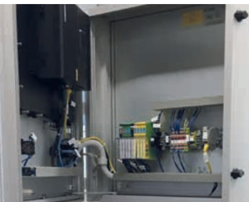
Assembly and wiring
